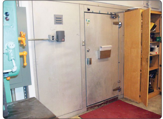
Figure 7-44. Walk-in freezer for storing prepreg materials.
