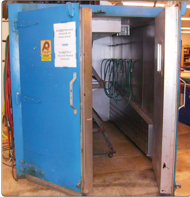
Figure 7-38. Walk-in curing oven.
